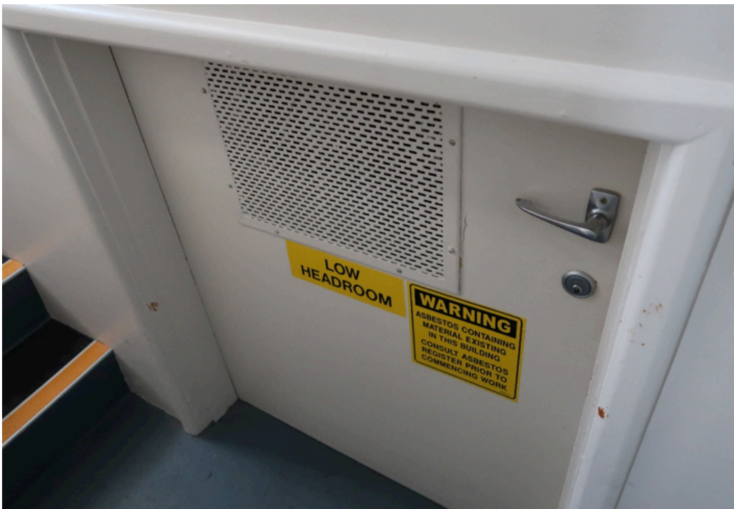
Figure 56 Door to the crawl space under the cabin: note asbestos 'warning' sign
