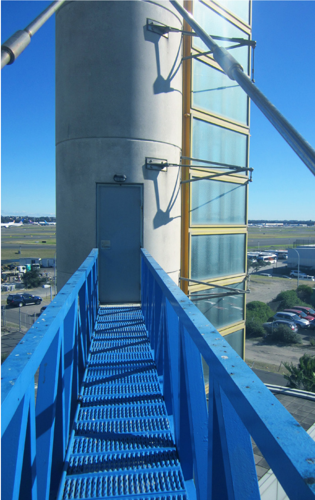
Figure 22 Two bridges provide access to the services riser within the concrete shaft
