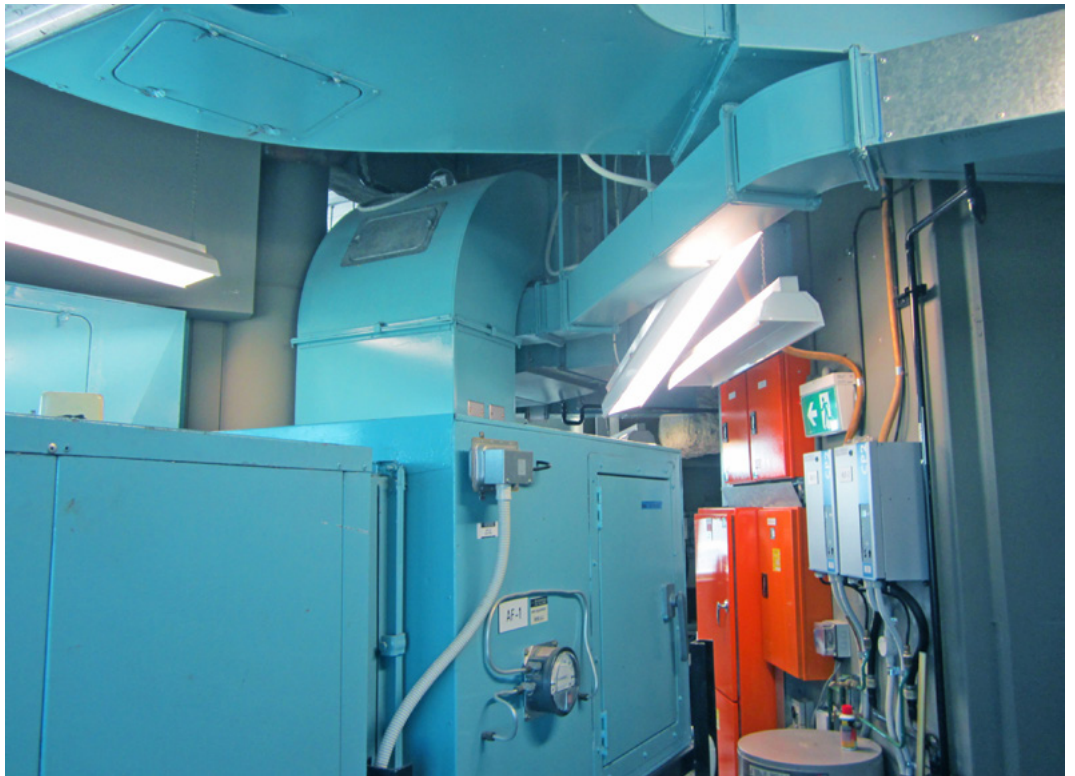
Figure 27 Air-conditioning plant on the amenities and plant room level
